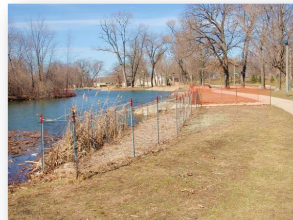
Temporary fencing to protect a park shoreline and newly-planted goose-resistant vegetation from wear and tear by geese
